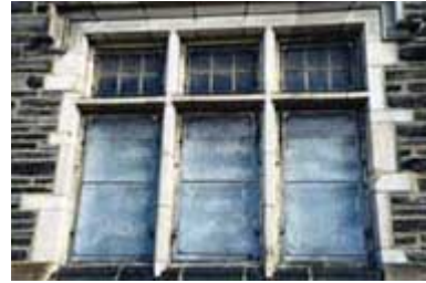
BEFORE: Example of deteriorated window conditions.
